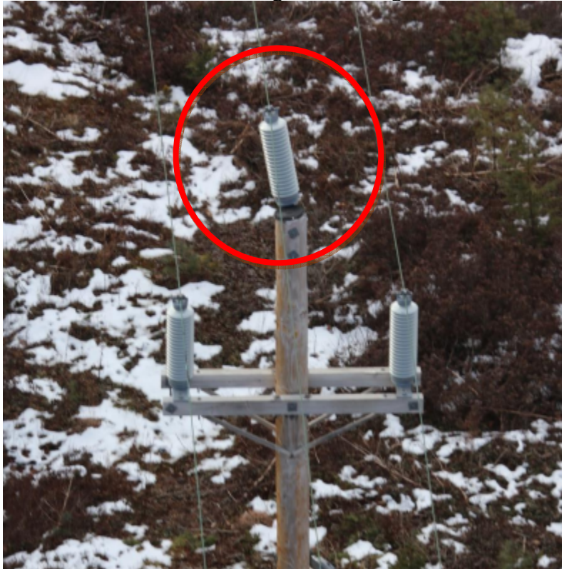
A1/B2 Structure 323-1 Damaged or leaning isolator
