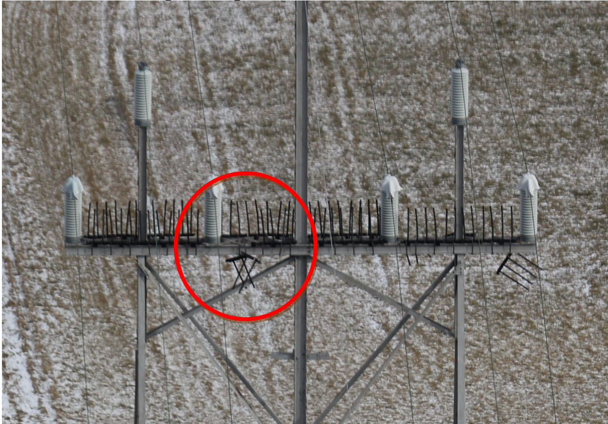
A1/B2 Structure 42 Damaged/Missing bird deterrents
