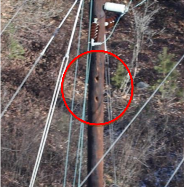
A1/B2 Structure 343-1 Woodpecker damage
