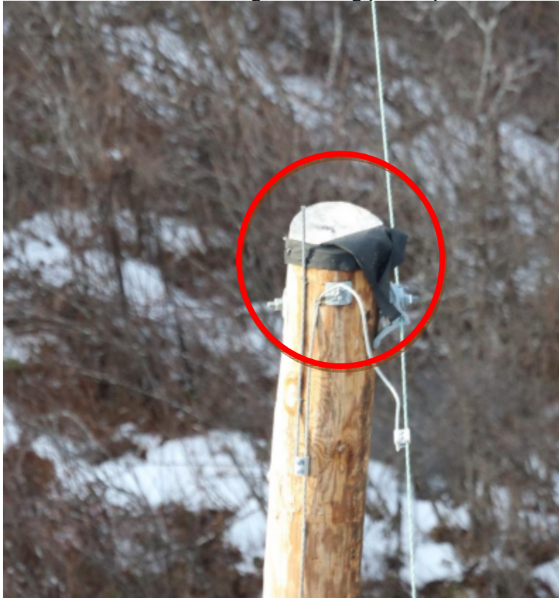
A1/B2 Structure 397 Damaged/Missing pole cap
