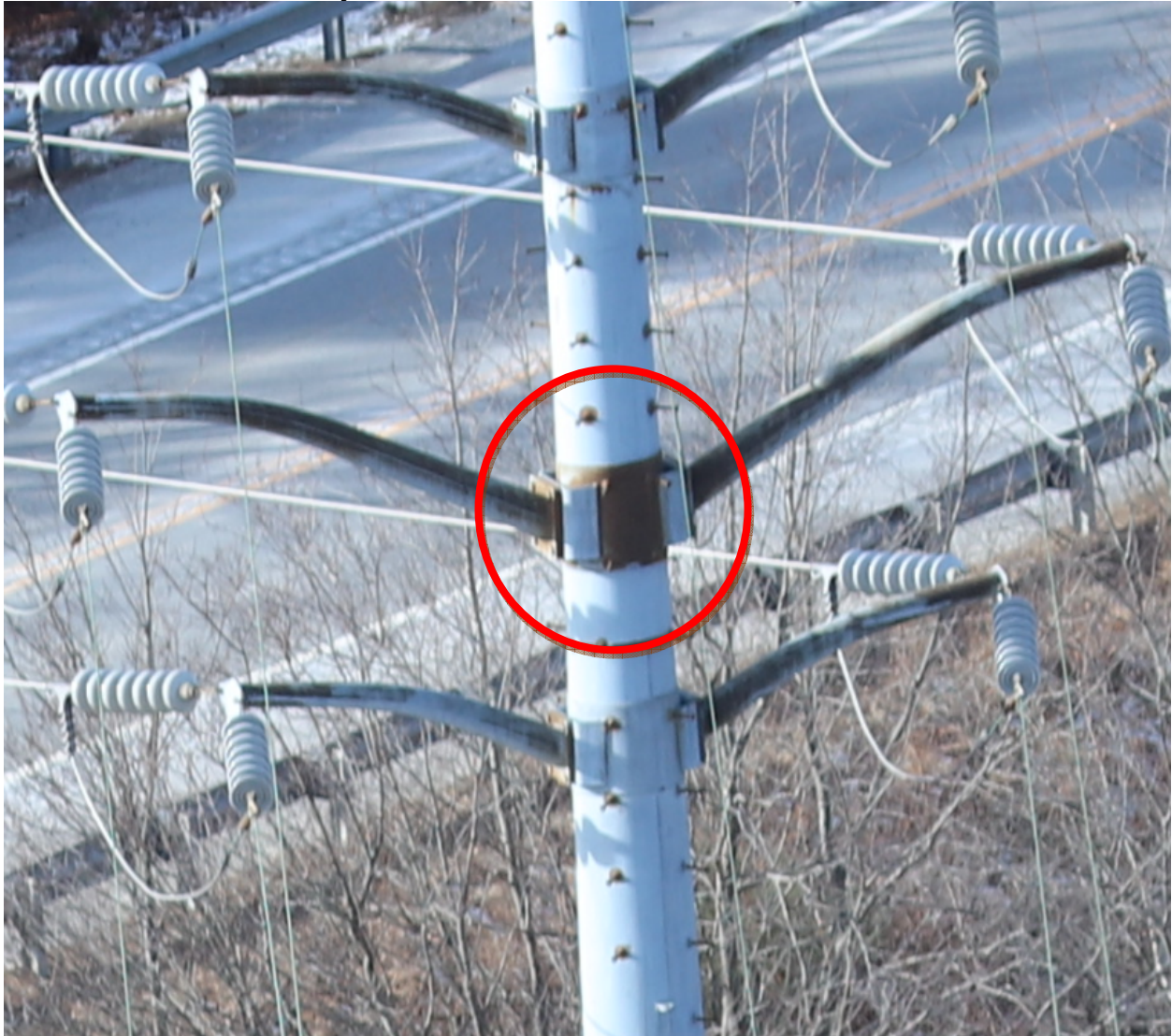
A1/B2 Structure 472-1 Rusty davit arm collar
