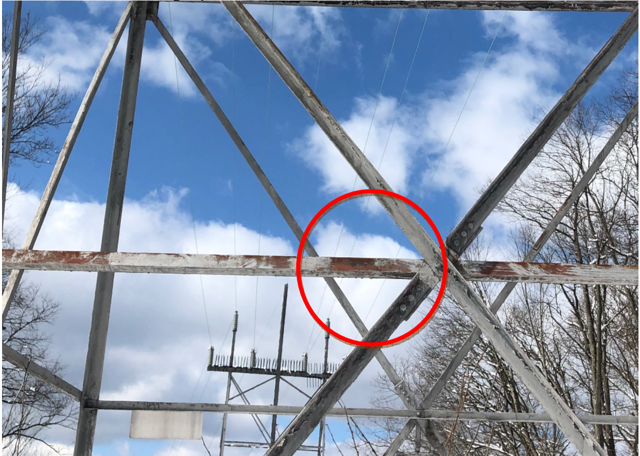
A1/B2 Structure 48 Damaged paint
